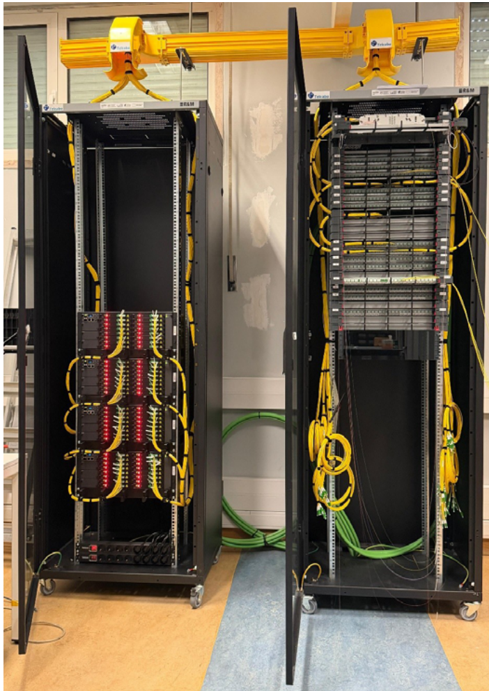
LUMIRing Hub: This image showcases the LCO cabinets, featuring access to the cores of MCFs on the right and optical amplifiers designed for long-haul transmission on the left.
